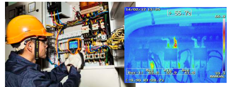
Predictive maintenance on electrical systems
