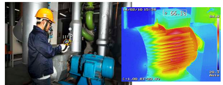
Predictive maintenance on electromechanical systems
